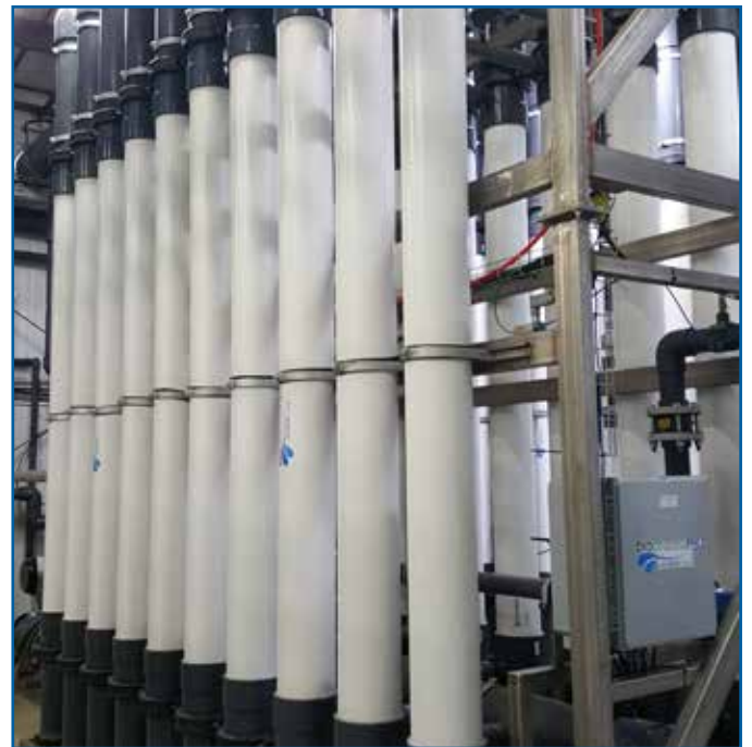
Pentair X-Flow Membrane Skid.
