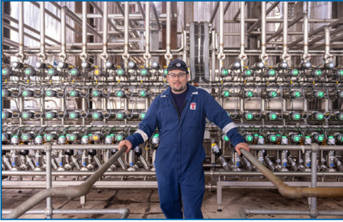
Alistair Fyfe of Tennent's Brewery standing in front of the Pentair Südmo Double Seat Valve Gas Manifold.
