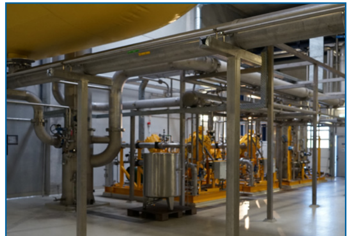
Pentair CO 2 recovery technology is also present at Paulaner Brewery.
